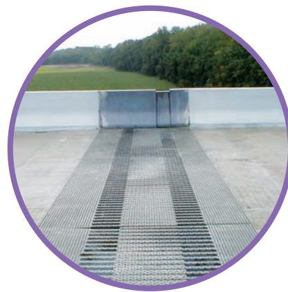
Figure 7.3C Highways and bridges must be built with gaps to allow the expansion of the pavement.
